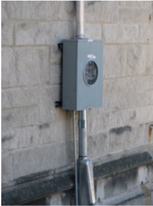
Figure 10 Temporary power box for electrical work waiting for ComEd review and approval.
