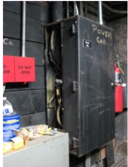
Figure 12 Church Building Power Panel showing damage to input cable. See cable damage above red box on large diameter leads.
