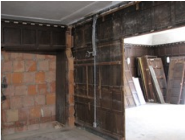
Figure 3 Aki's Place area. most of CM Parlor/ Aki's wall removed. Old storage area
