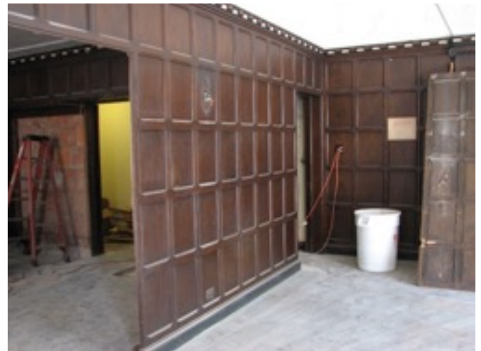
Figure 5 CM Parlor & Aki's Place. Remaining wood panels will be opened, leaving only two panel sets top to bottom. Rest of opening will use new folding doors.
