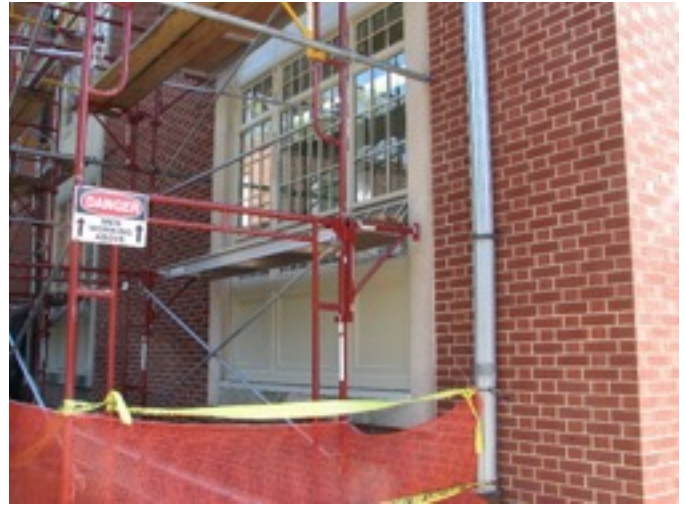
Figure 8 North wall Pennington Center. Scaffolding is expected to be removed at end of October.
