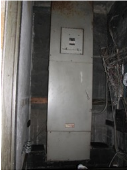
Figure 13 Separate Pennington Center Power Panel installed in 1962. This too will be replaced.
