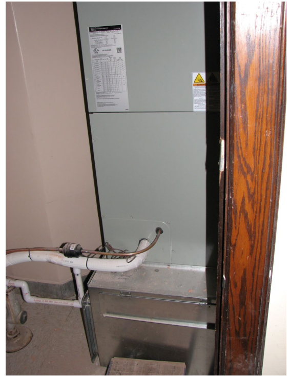
Figure 9. AC in old Parish House Janitor's Closet.
