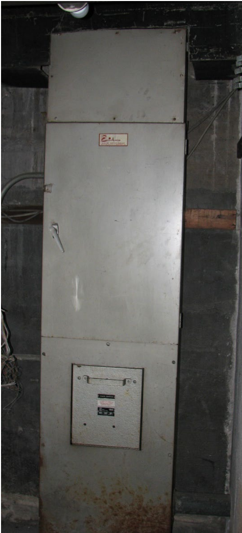
Figure 12. Pennington Power Panel (~1963).
